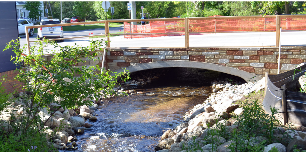
A new bridge over Kids Creek at the Seventh Street entrance to the Emergency Department completes creek restoration efforts on MMC's campus.
