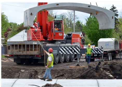
A Traverse City worker guides a piece of bridge for Kids Creek into place.
