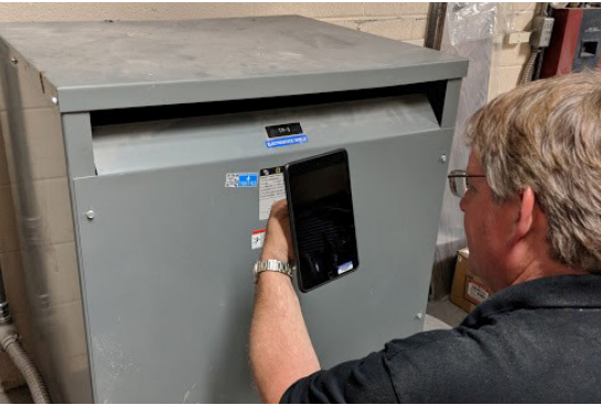
Charlevoix Hospital Maintenance Director Bruce Giem scans the asset bar code to add the equipment into the eMediTrack system.
